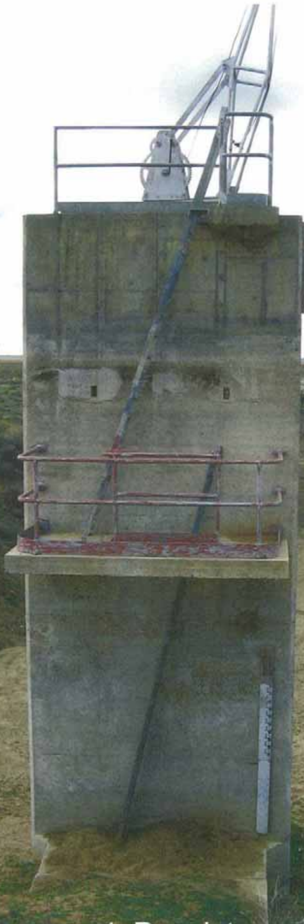
4. Regulator on empty Lake Cawndilla - note water levels near top of tower
